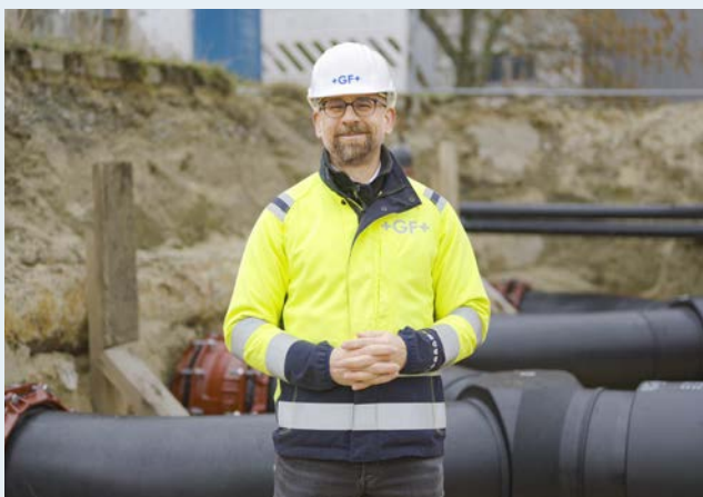
GF Piping Systems’ Fabian Probe, Technical Manager for Infrastructure (Germany), was on-site, supporting the installation of GF’s flow solutions, including GF’s BIG couplers and MultiJoints.
